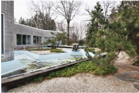
Rebuilt pools, having failed again, along with overgrown plantings beside the path of the EarthCam building, 2014 - Photo courtesy of EarthCam
