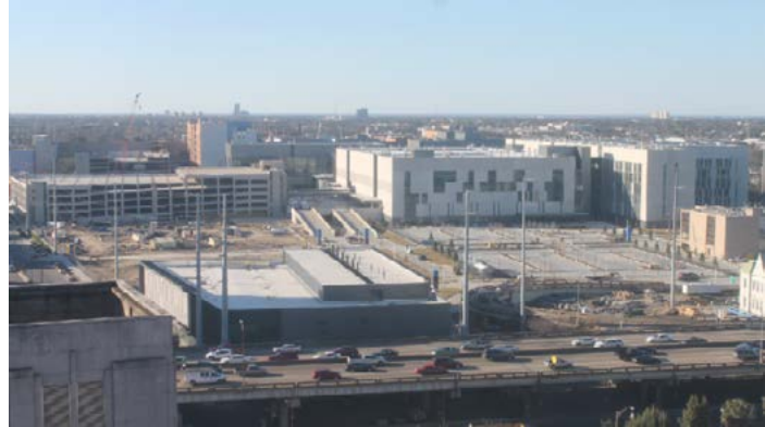
A March 10, 2015, screen capture from earthcam.com shows construction progress on University Medical Center. The hospital has a new target opening date of Aug. 1, a spokeswoman said. ( Earthcam.com and Interim LSU Hospital)
