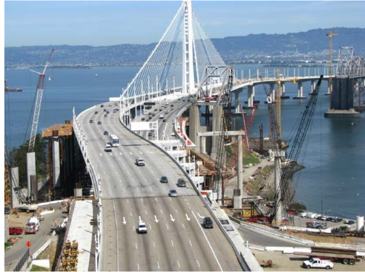
EarthCam is proud to support the engineers and construction teams by documenting the progress of the San Francisco-Oakland Bay Bridge.
