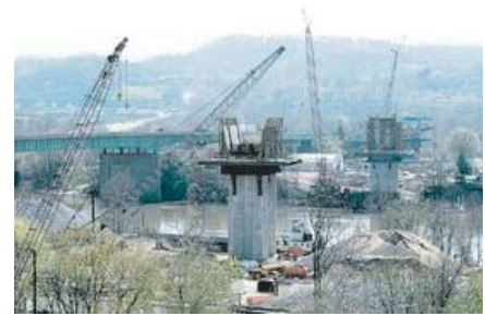
Five of the seven piers have been erected to support the new Interstate 64 bridge connecting Dunbar and South Charleston. Crews anticipate the bridge to be completed in late 2010.
