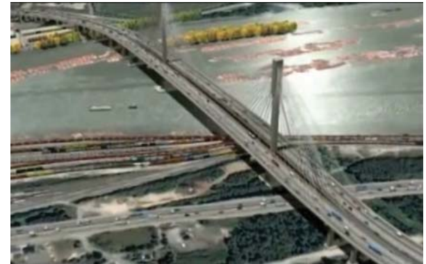
Construction of the CA$ 2.5 billion Port Mann Bridge over the Fraser River in the Province of British Columbia, Canada has started. The bridge will have 10-lanes and replace the existing crossing instead of standing alongside it.
