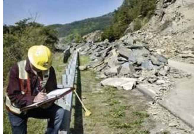
In this recent photo, Lewis Clarke takes notes about recovery efforts under way at the site of a rockslide that has closed The Dragon on U.S. 129 in Blount County.
