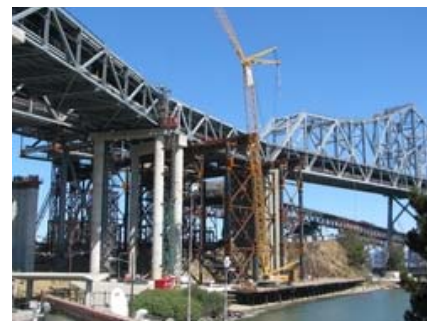
An EarthCam camera view of San Francisco Bay Bridge seismic retrofit project
