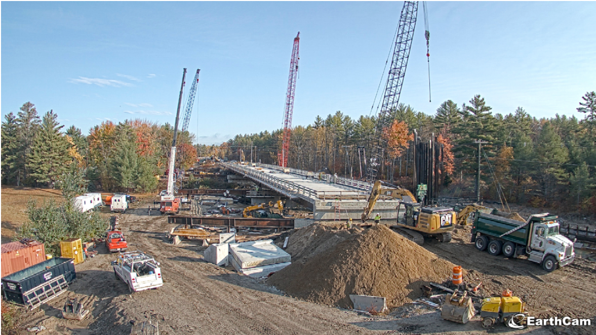
Reed & Reed crews slid in the new bridge after demolishing the old one within 84 hours as part of the New Hampshire Department of Transportation's first bridge-slide project.
